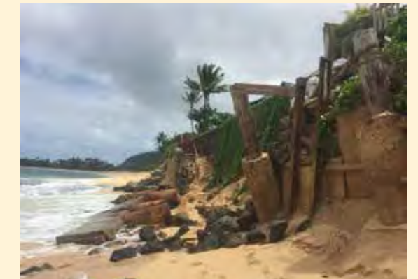
Failed and encroaching sea walls along the North Shore
